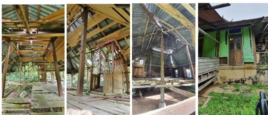
Figure 2: The deteriorating condition of timber structural elements.
