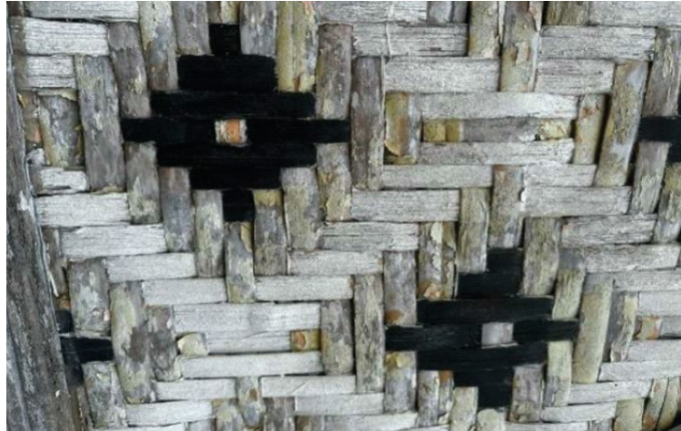
Figure 1.0: Current condition of the Kelarai walls of Ihsaniah Iskandariah Mosque, Padang Rengas (Source: Syed Mustapa et al., 2024)
