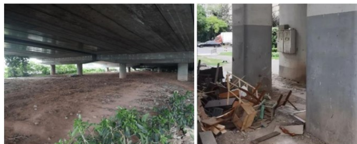
Figure 2: The Space Under the Bridge is Disorderly and the Utilization Rate is Low Source: Photographed by the author (2024)
