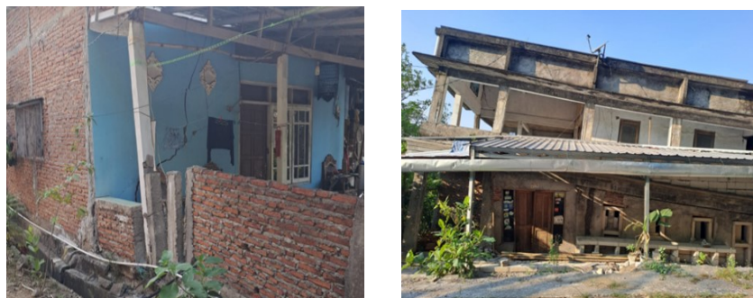
Figure 4. Figure of the damaged house caused by slow and sudden landslides in Sukorejo Village, Gunung Pati District.
